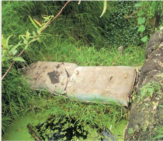
FIGURE 53. Simple costalera installed to prevent water from flowing too rapidly towards the northern part of the zone, which has become lower as a result of differential subsidence.
